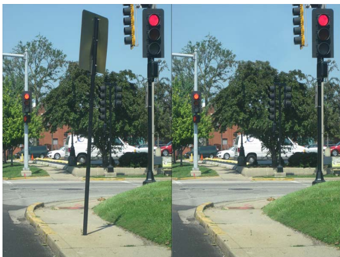
Poor sign placement forces users onto street or grassy bank
